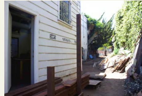
2021: The space is cleared out and a door from our center to the back yard is built.
